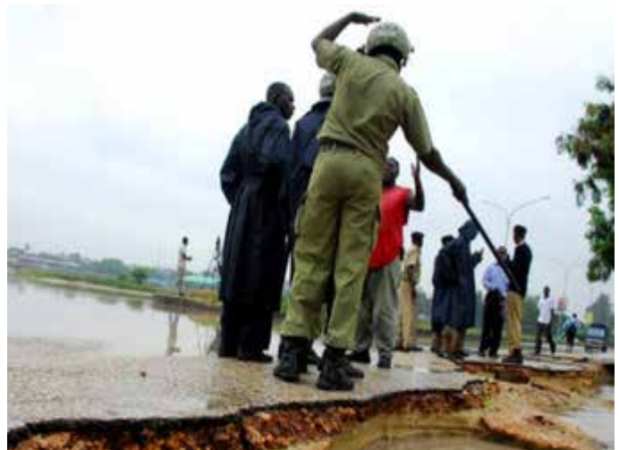
Plate 2: Tanzanian police officers inspect part of the damaged road in Dar es Salaam in 12 th April, 2014. (Deodatus Balile /Sabahi)
