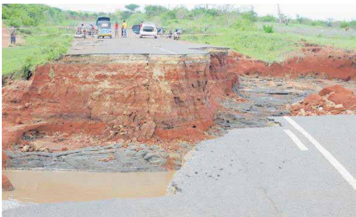
Figure 11: The Handeni/Korogwe road section was washed away following the ongoing heavy rains at Sindeni in Handeni District in Tanga Region on Saturday 26 th October 2019 (Source https://www.thecitizen.co.tz/news/1840340-5328818-9slyoo/index.html )
