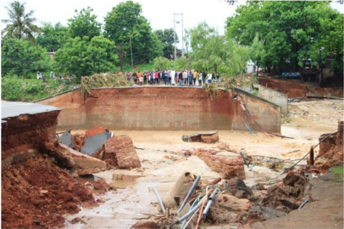
Figure 2: The bridge connecting Kunduchi and Bahari beach being damaged and broken after heavy rains (Source: Mwananchi newspaper).
